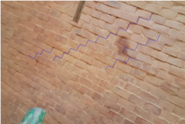
Shear cracks and settlement of the squinches
