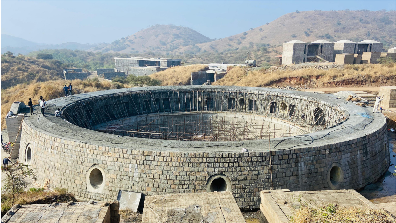
Stone wall construction with specially fabricated template, integrating customised formworks for conical windows
