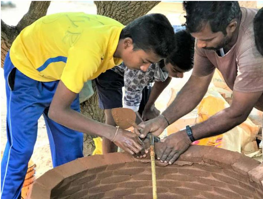
Students from Udavi School learning to use the compass for dome construction
