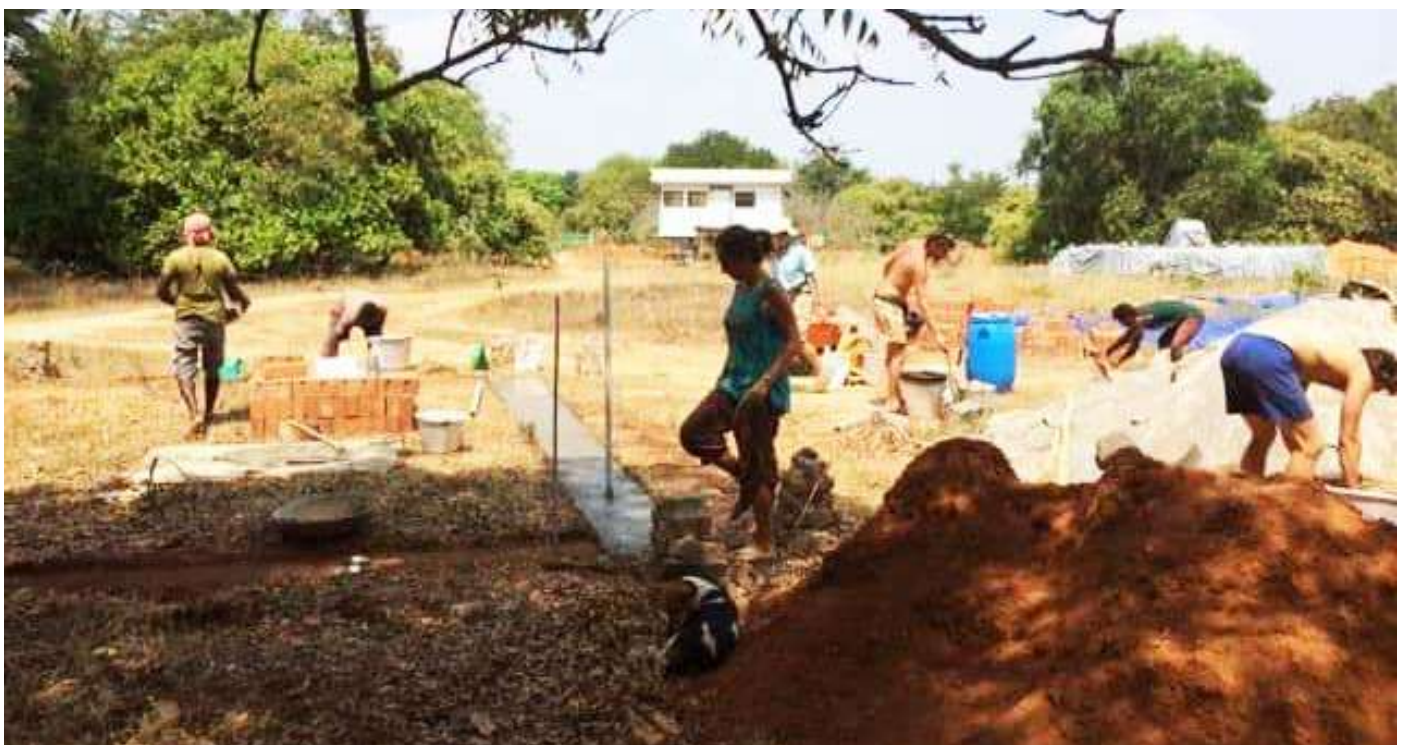
Work beginning on the social space, which will be constructed with poured earth concrete, at Joy of Impermanence
