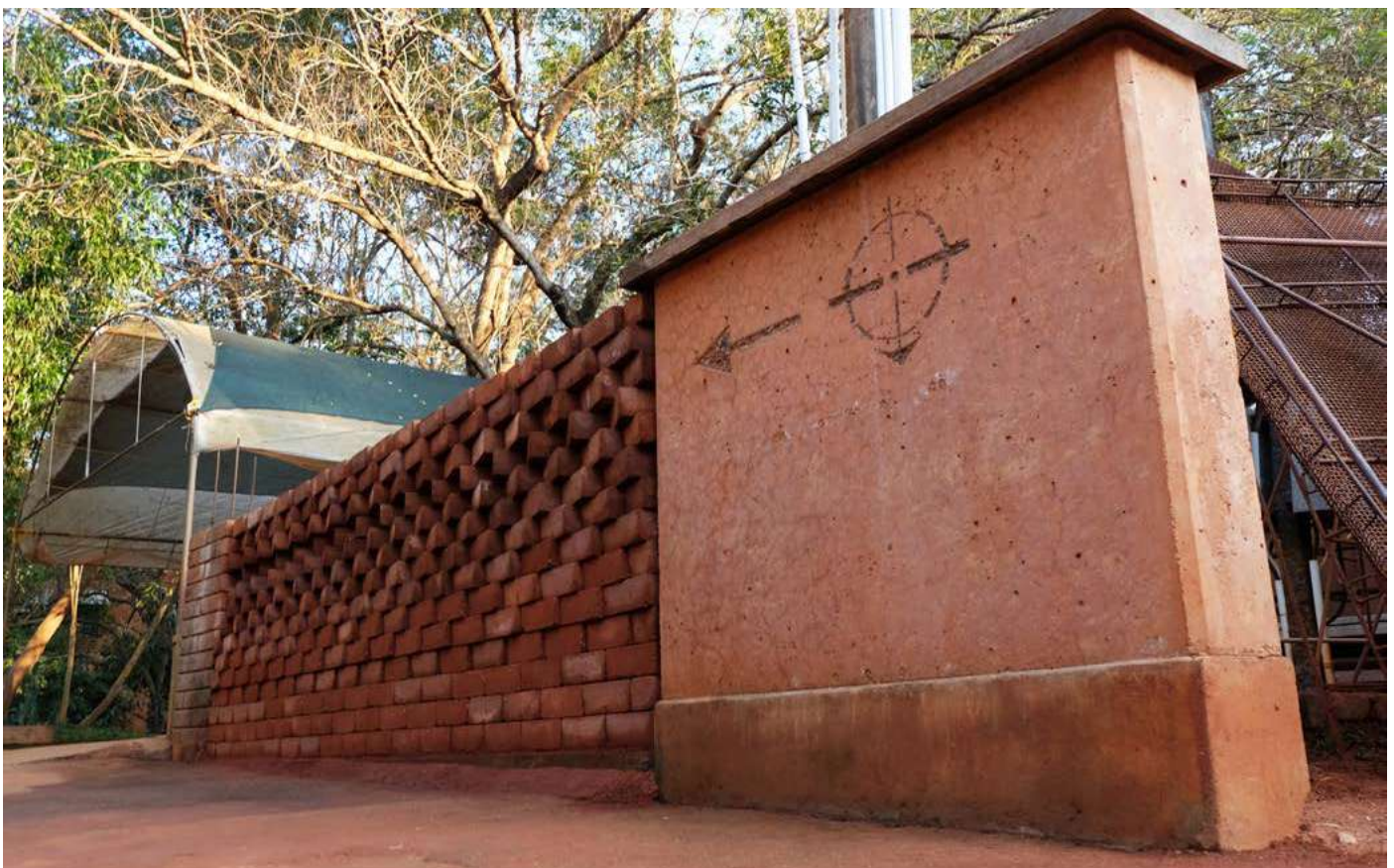
A dry laid CSEB wall and carved poured earth concrete done by Lara for the AVEI Open House
