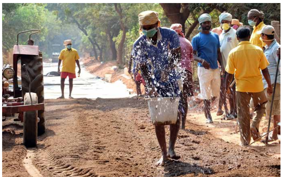
Road Service at work on the Stabilized Earth Concrete road, with assistance from Satprem, Ayyappan, and the rest of the Earth Institute team
