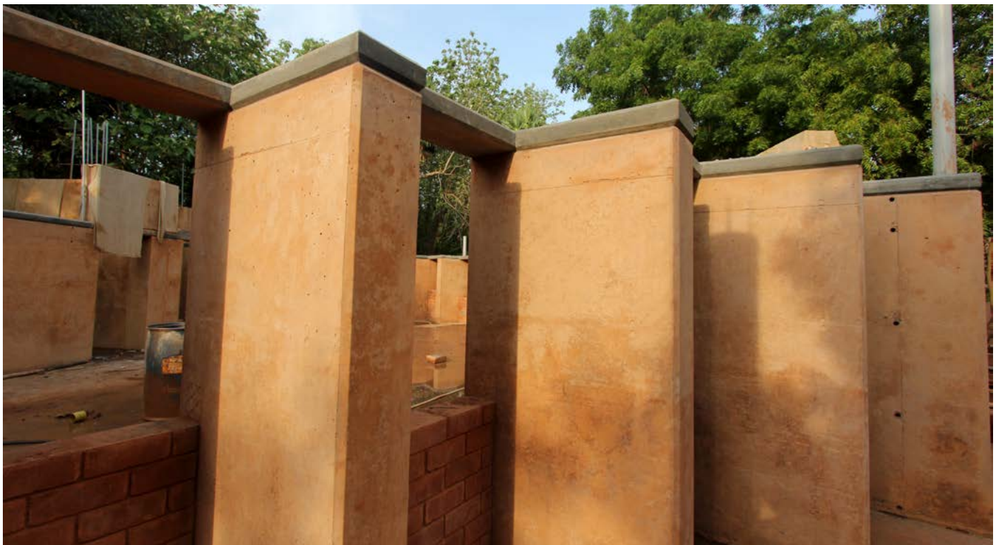
A sneak preview of the Conference Hall currently under construction... vault construction will begin soon!
