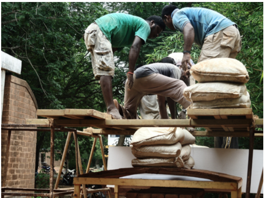
Laying the first layer of bricks with the free-spanning technique ; The second layer with rotated bond pattern ; Load testing the vault
