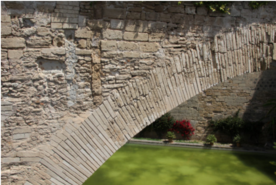
Royal Palace of l'Almudaina, Mallorca - Fortified rammed earth structure clad in stone
