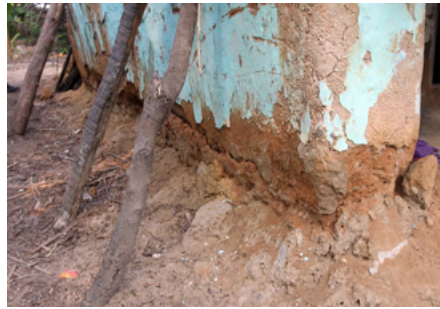
Capillary erosion and wall tilting
