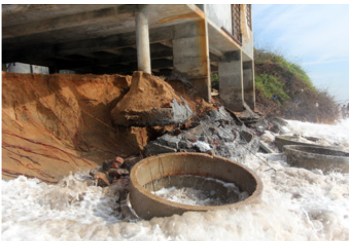
Exposed foundation at Philippe's house
